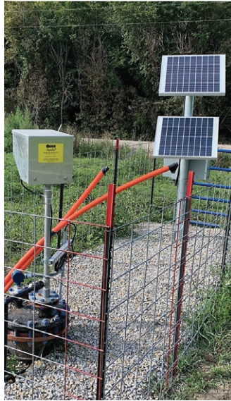
Solar-powered Apollo, pumping methane biogas condensate sump at large Midwest bioenergy operation.
