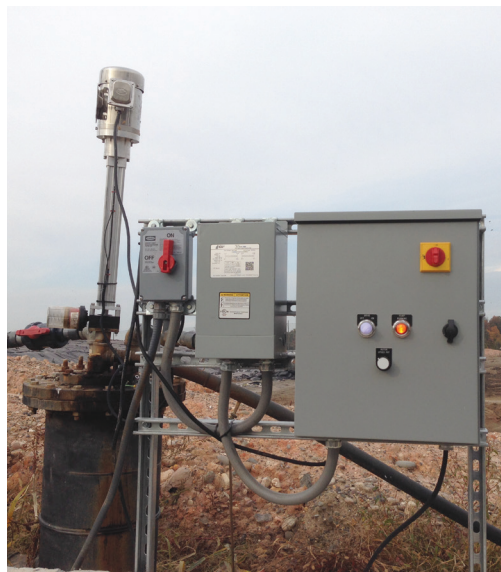
Anchor pump with control panel
